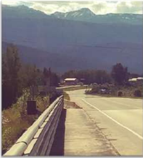
Figure 13: Fraser River Bridge - barricades blocking users on shoulder from accessing sidewalk (looking westward)
