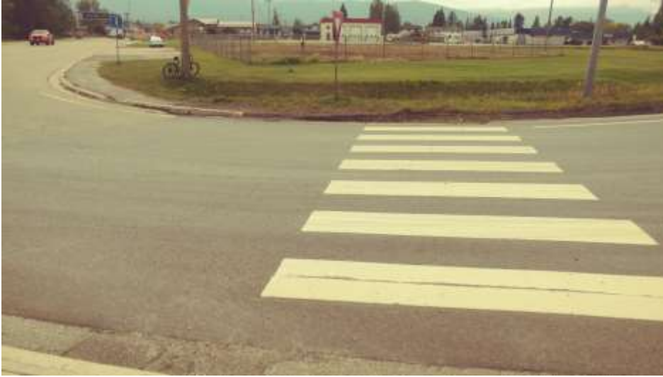
Figure 4: Missing portion of sidewalk at NW corner of Highway 16/Main St. Intersection
